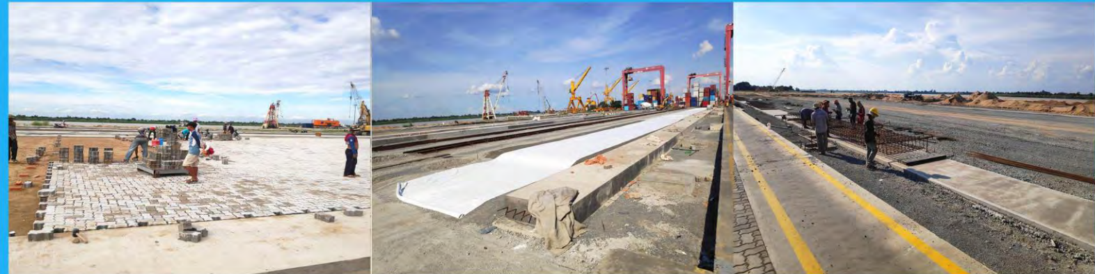
Construction of RTG lanes and concrete block yards for Phase III Expansion of the Container Yard.
